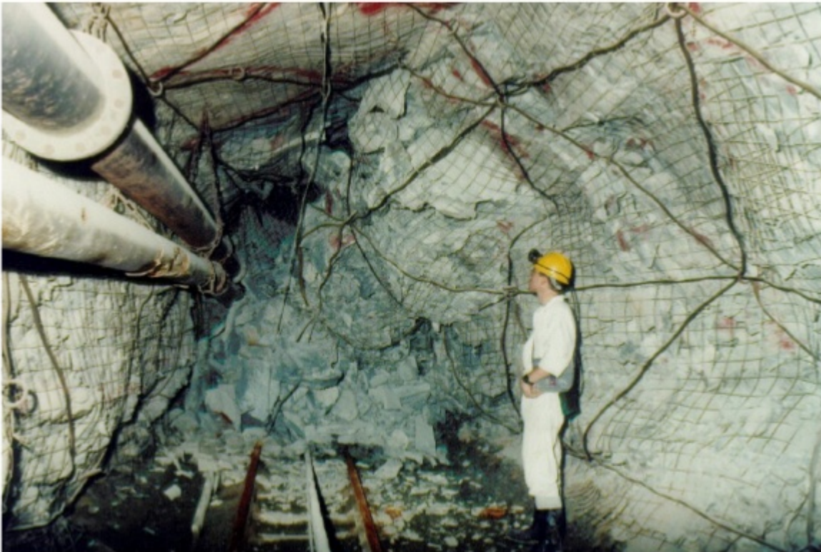
Aftermath of a rockburst in a deep-level tunnel showing complete tunnel closure. The energy released by this event is equivalent to magnitude M = 3.4 earthquake .
